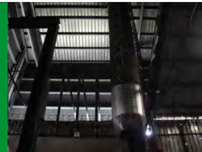
Steam boilers with no heat recycling systems
